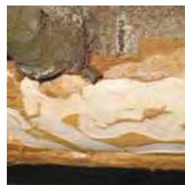
Boring galleries underneath bark
